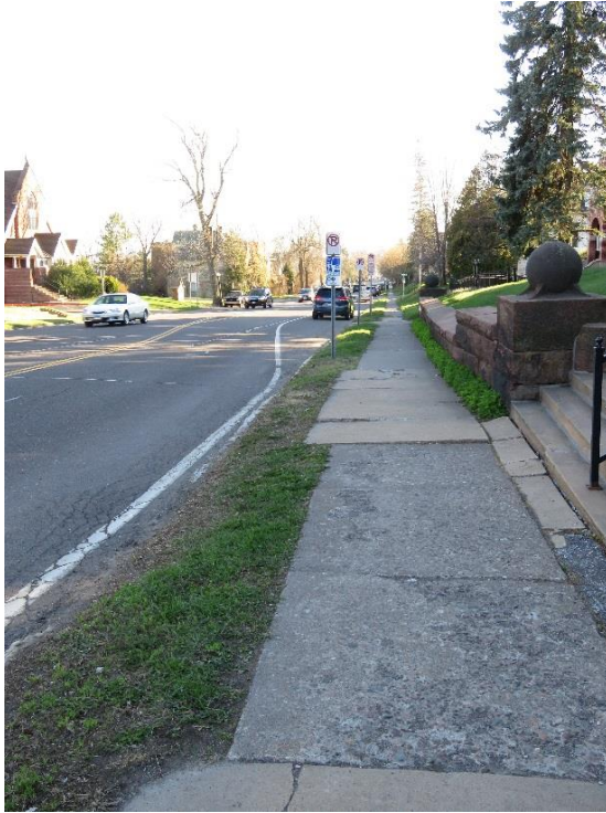
Deteriorated sidewalk adjacent to bus stop
